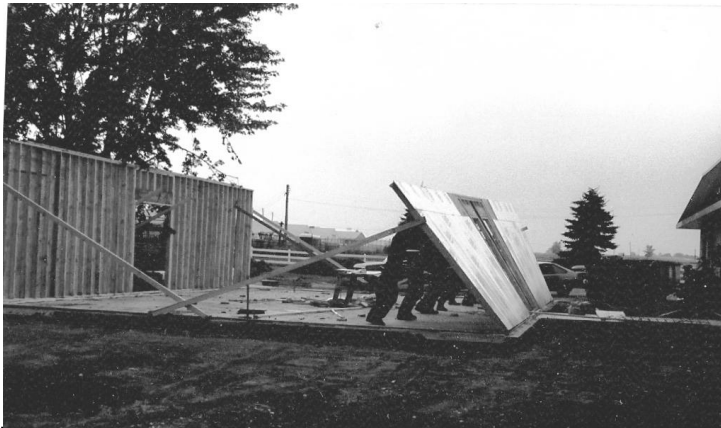
Workers raise the walls on the KCFB auditorium in this 1986 file photo.
